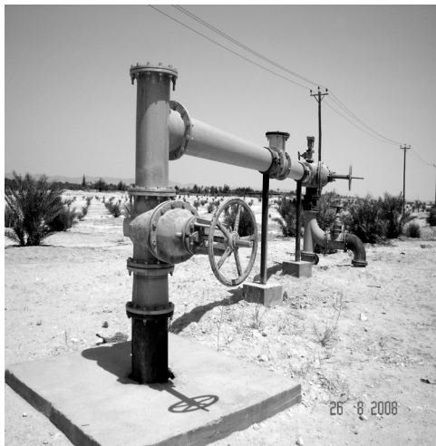
Figure 1. Well head of existing geothermal source
